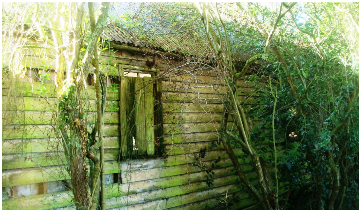
Picture 8: The late 19 th century Mission Hall building now in a state of decline Officers would welcome discussion with the owner.
